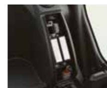
Central fuse box located behind seat
