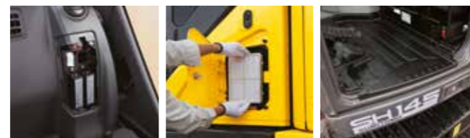
Central fuse box located behind seat
